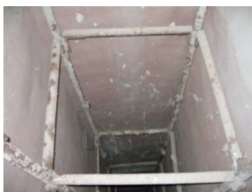
The Lift Shaft – sadly still in the same condition!
